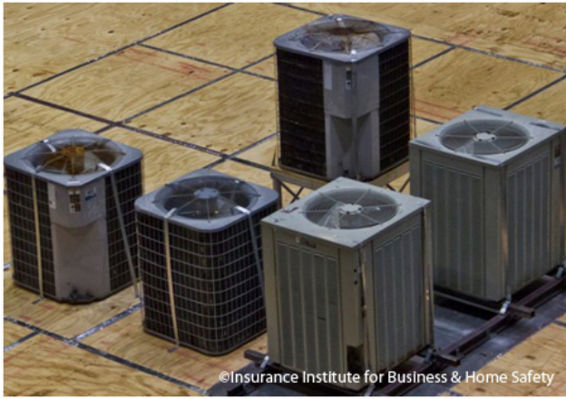
Secure AC units like those shown above in order to reduce the risk of damage to the equipment during high winds.
